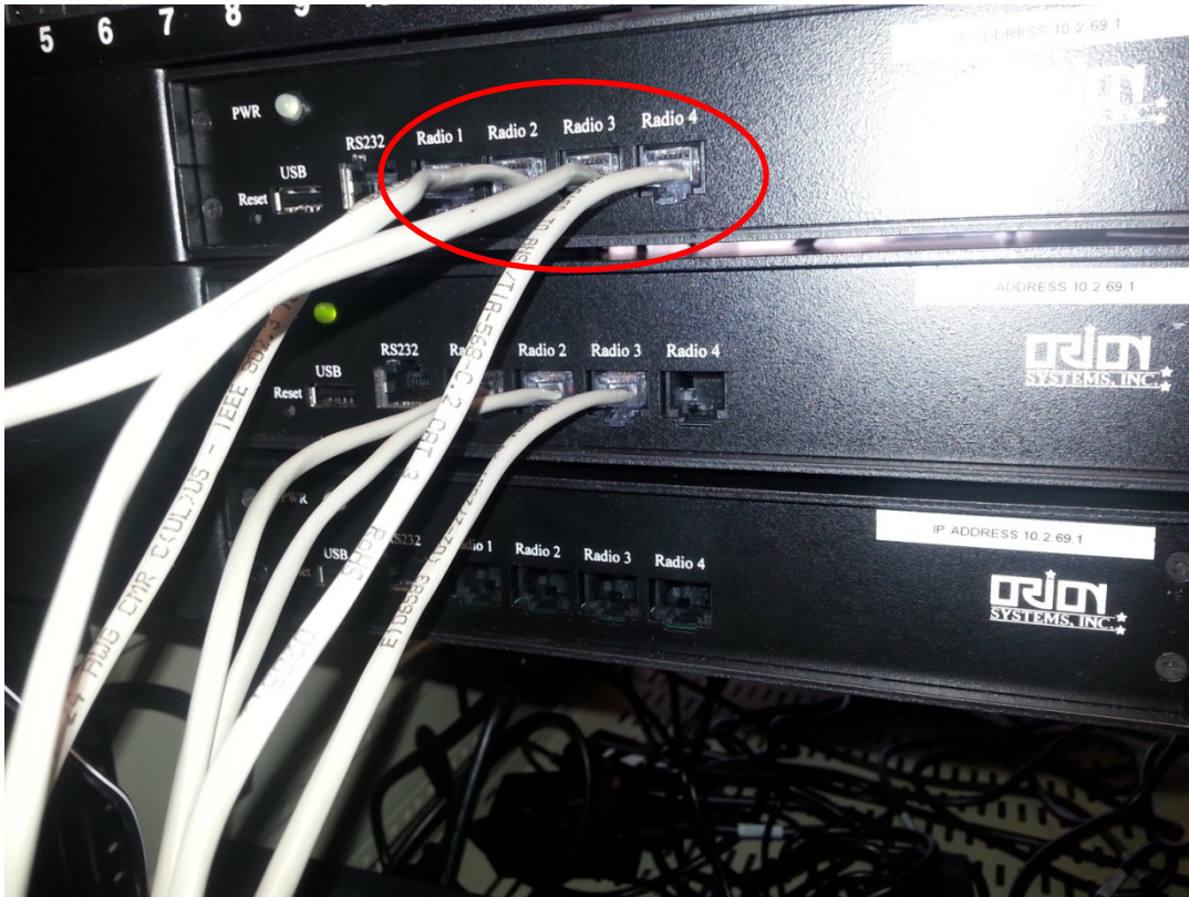
Exhibit 32.6-9 Connections to transmitters from failed DAC
