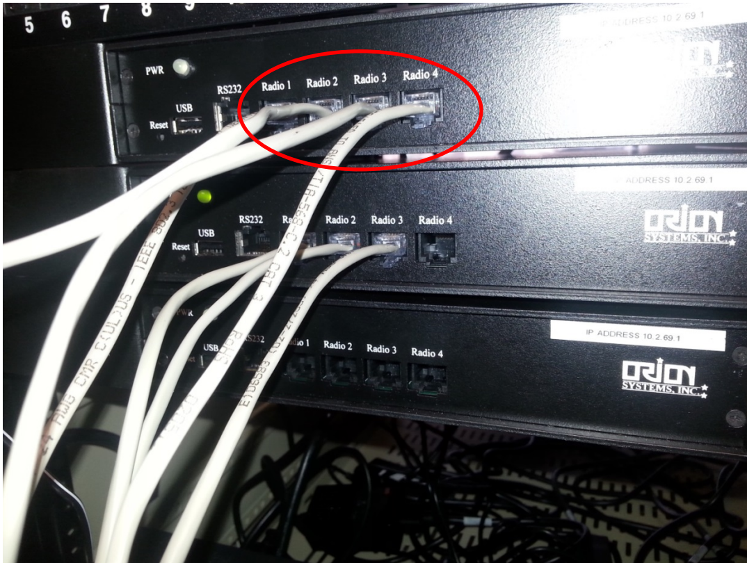
Exhibit 32.6-9 Connections to transmitters from failed DAC
