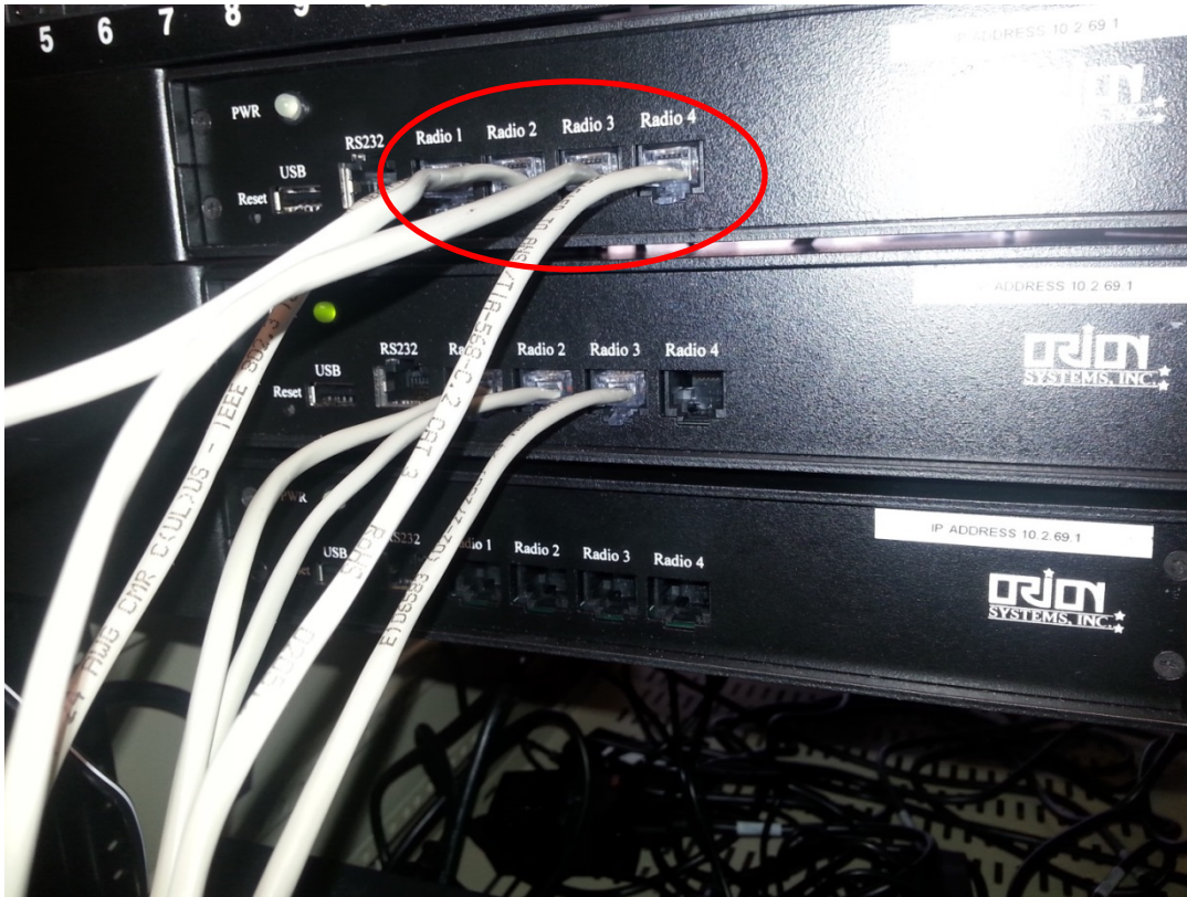
Exhibit 32.6-9 Connections to transmitters from failed DAC
